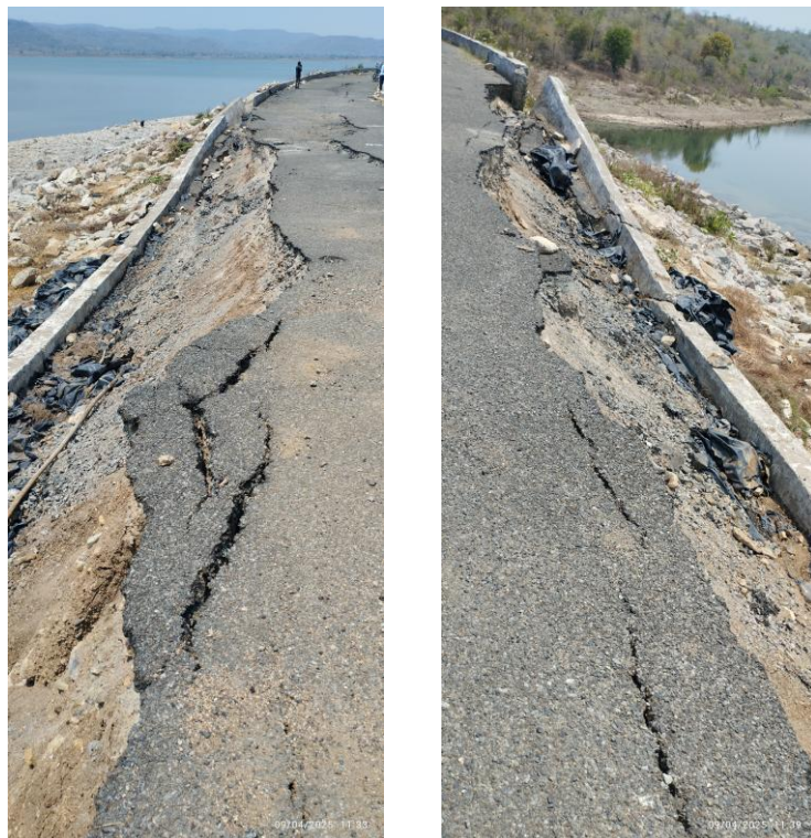
Figure 2.3 Slides in earthen dam
