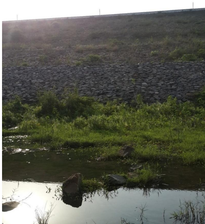
Figure 4.2 Seepage near downstream toe of earthen dam
