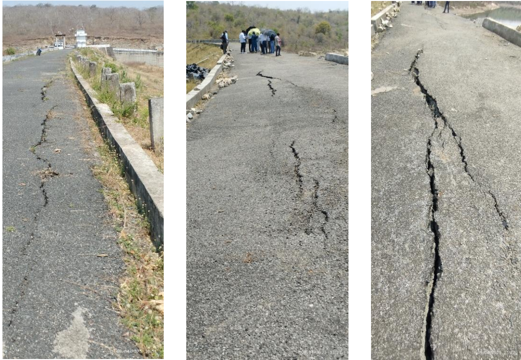
Figure 2.2 Cracking in earthen dam
