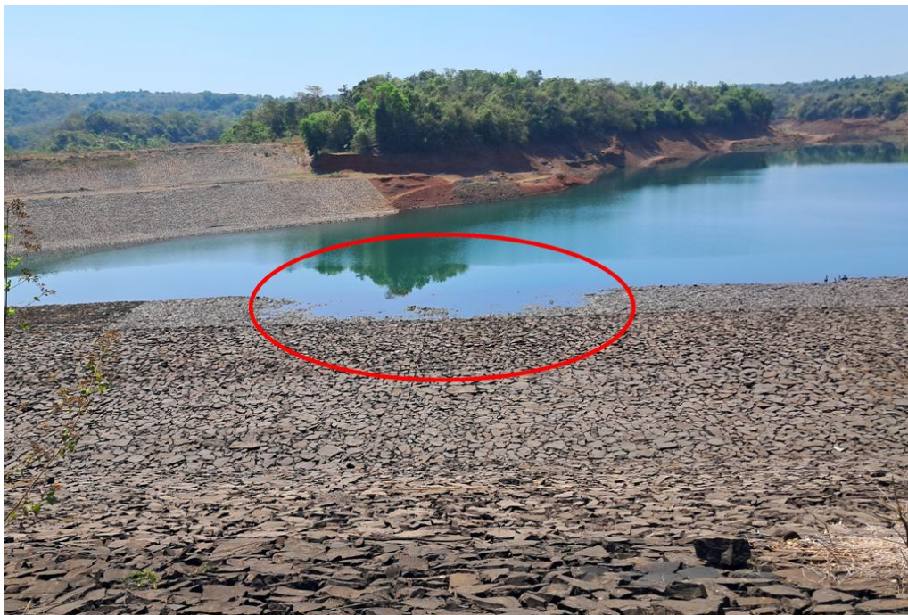
Figure 2.4 Indication of upstream berm settlement
